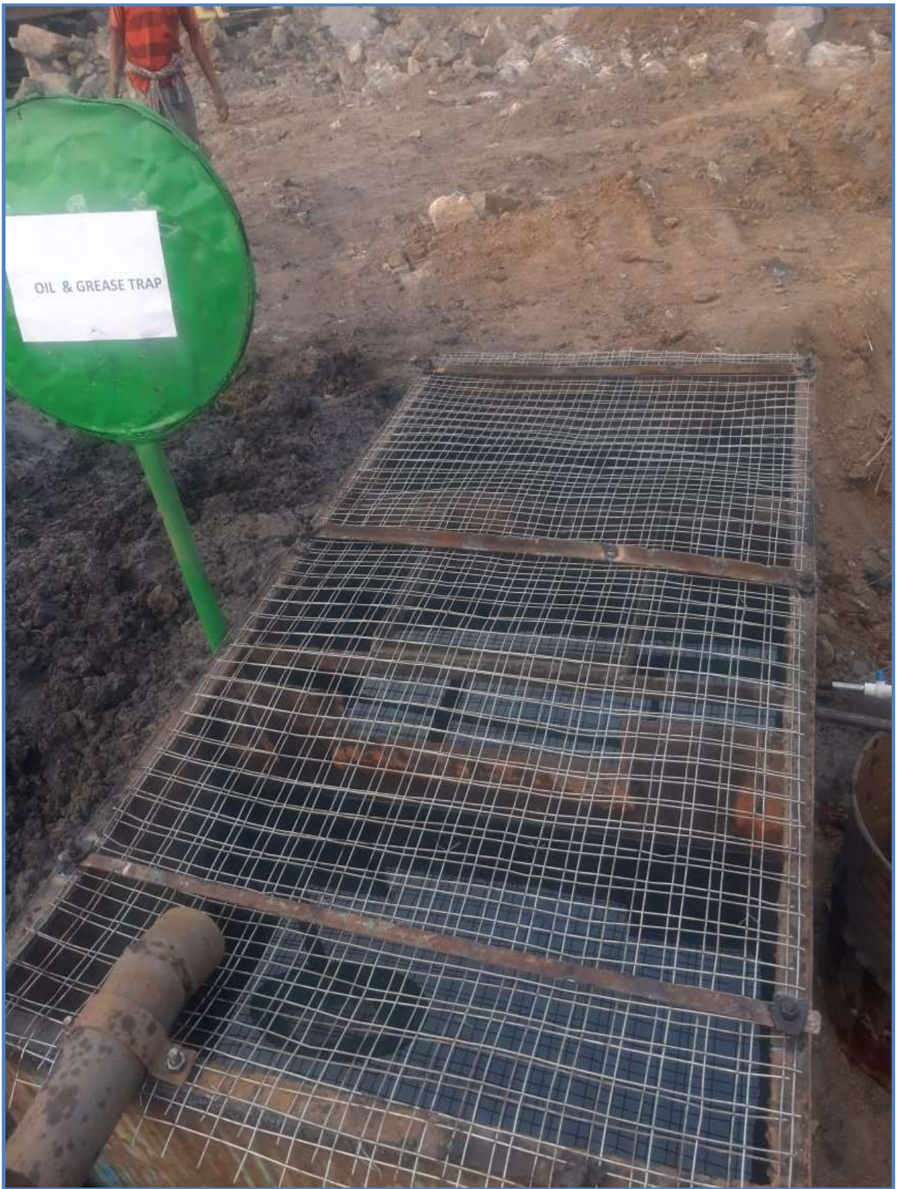
Picture 7 – Oil & Grease Trap
